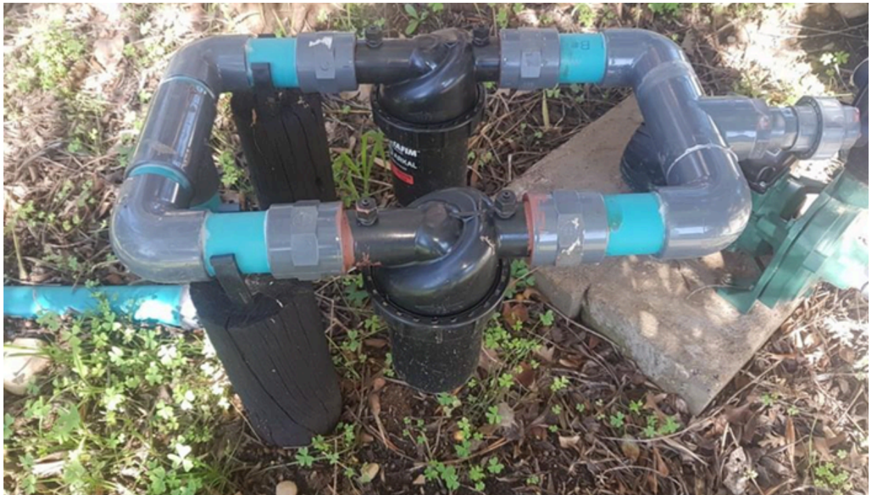
Figure 18. An image of the two-ring filters installed in parallel after the new pump.
