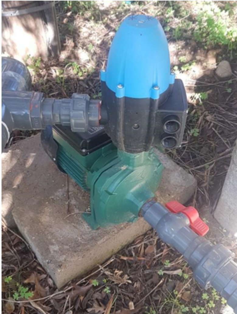
Figure 16. An image of the installed 0.37 kW DAB pump with fitted flow switch fixed onto concrete on Welgevallen Experimental farm.
